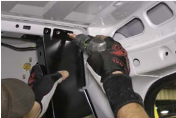
Roof rib holes
