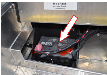
Battery Under the Stepwell Lid
